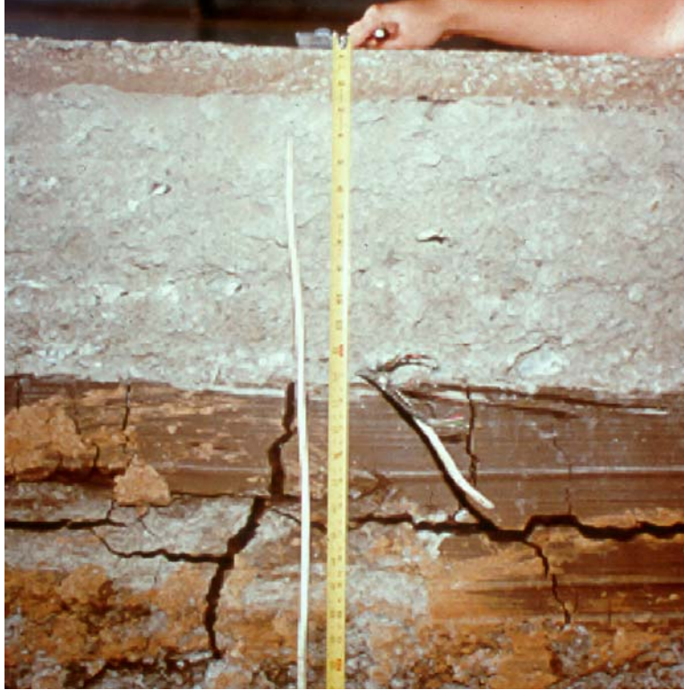
FIGURE 1 Shrinkage Cracks in High PI Clay Covered by Lime-Treated Layer (Courtesy of Lytton and Freeman at Texas Transportation Institute).
