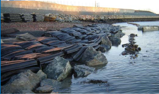
This Massachusetts shoreline is now protected against severe erosion caused by weather and waves.
