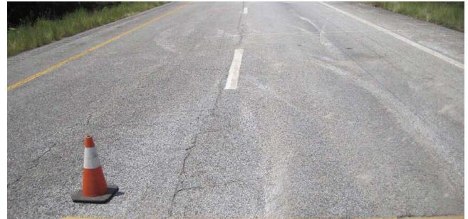
During the 2018 site visit, additional cracking was observed in the unreinforced section.
