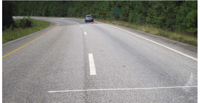
The GlasGrid reinforced section was also evaluated in 2018. After 60 million ESALs, cracking was starting to appear but limited to the 18 yr. old construction joint.
