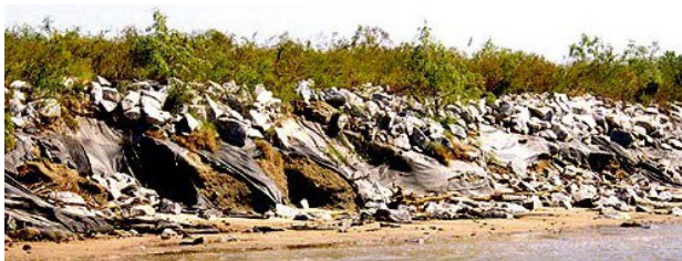
Figure 4: Close-up view of riprap failure at Section E.
