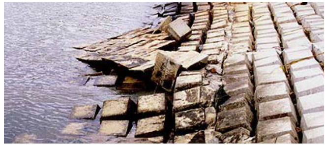
Figure 13: Flipping of cabled block mat on the upstream portion of Section A.
