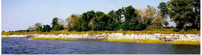
Figure 5: Downstream portion of riprap Section G. This section experienced three distinct failed areas. Left is upstream, right is downstream.
