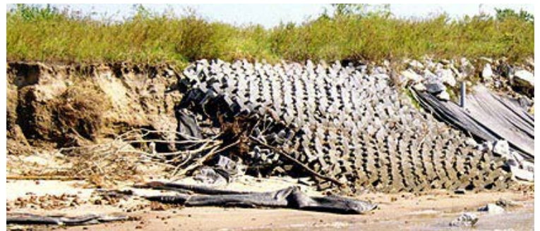
Figure 14: Washout of tetrapod units at upstream flanking of Section E. Upstream edge is undermined and generally not flexing with the subgrade.
