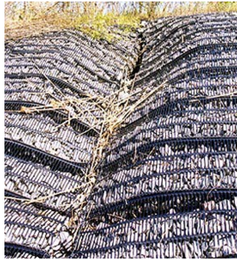
Fig. 21: A void two to three feet wide and two to three feet deep had developed beneath two units and near the top of the slope. Video inspection of the void showed that the geotextile underlayer was missing and apparently had not been placed. The upper edge of the geotextile was found at the lower end of the visible gap (the top third of this photograph). The void had propagated downslope.
