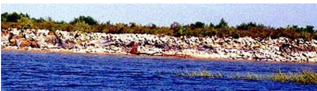
Figure 3: Upstream portion of riprap installation at Section E. This area experienced major washouts.
