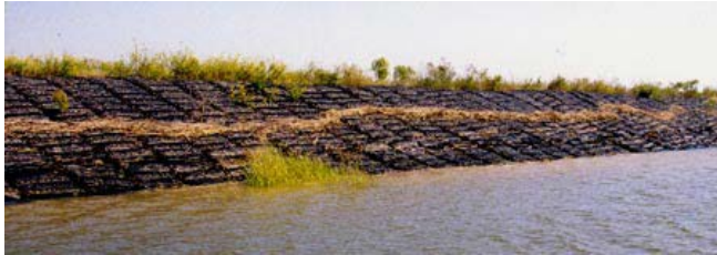
Fig. 17: Marine mattress Section C looking downstream. Each unit is anchored at top of slope by burying an extending tail of geogrid. Pairs of units are spliced together end to end. Stability has been maintained throughout.
