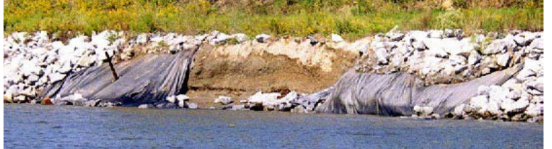
Figure 6: First (upstream) failed area at riprap Section G
