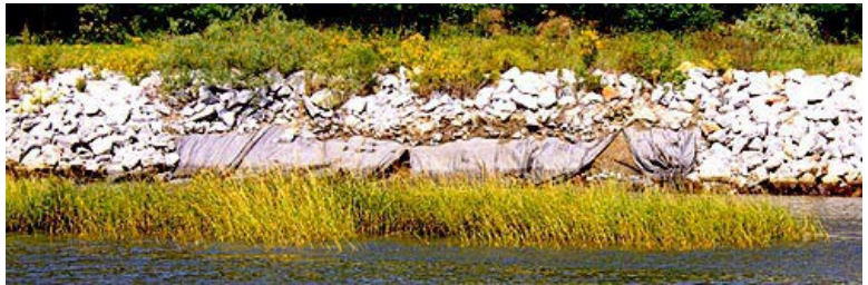
Figure 7: Second failed area at riprap Section G.
