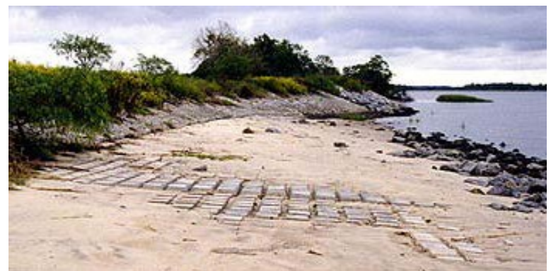
Figure 9: Cabled block mat Section D looking downstream. This site has been depositional, as evidenced by the sand deposits covering the armor layer.
