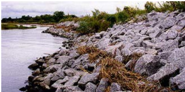
Figure 2: Riprap installation at Section B. In the vicinity of the vegetation in the center of the photo, slumping continues despite repairs by adding riprap.
