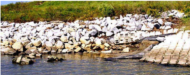
Figure 11: Cabled block mat washout at the flanking transition on the upstream end of Section A.
