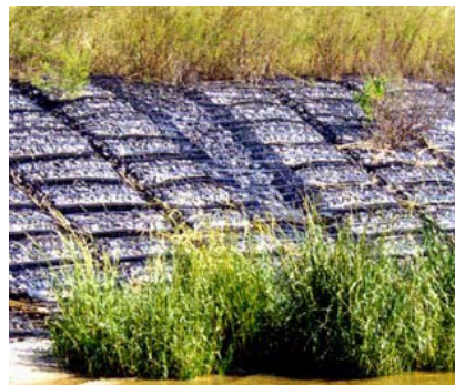
Fig. 20: An excessively wide gap at the side-to-side joint between marine mattress units has been repaired by filling the gap with stone and braiding a geogrid patch in place over the stone. Lesson learned: due to the excessive width of the gap, baffles are needed to prevent movement of stone down the slope.
