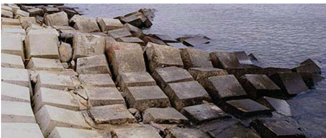
Figure 12: Heaving of cabled block mat on the upstream portion of Section A.
