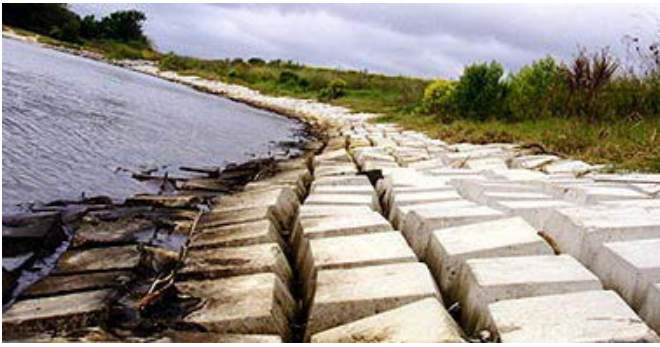
Figure 10: Cabled block mat Section A looking upstream. This site has been erosional. Differential settlement and loss of intimate contact are prevalent.
