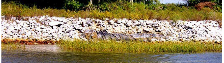
Figure 8: Third failed area at riprap Section G.
