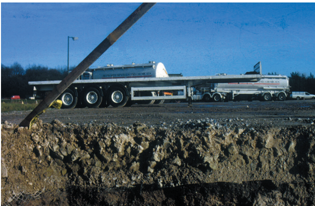
After 11 years of traffic in a truck parking area, the boundary between the base and subgrade remains distinct. Tensar Geogrid is the only material used to separate the base and the subgrade.
