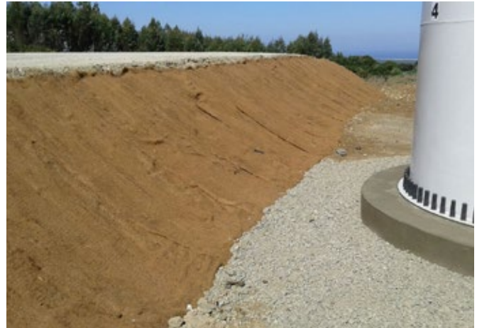
North American Green® EroNet® C125™ on a crane access road slope will provide erosion protection and vegetation establishment
