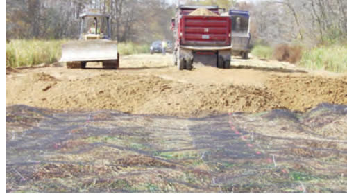
TriAx Geogrid created an unyielding and stable platform for constructing the berm.
