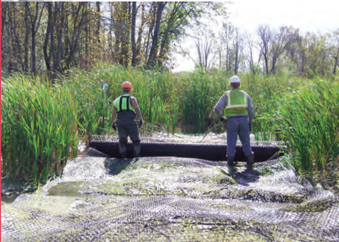
A layer of Tensar ® TriAx ® Geogrid was placed directly at the base of the berm to bridge the lake sediment.
