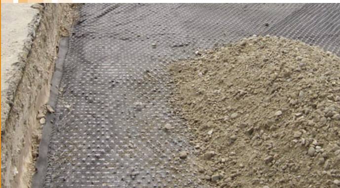
The Spectra® System delivered an affordable option to a site with challenging soil conditions.
