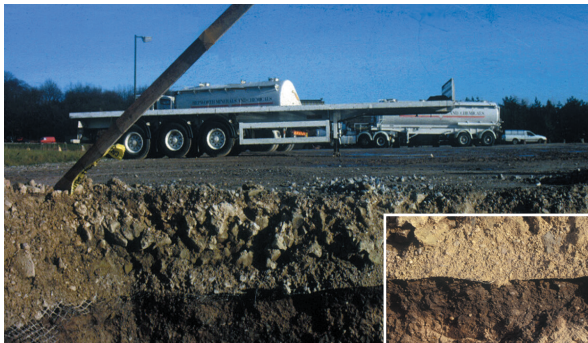
The boundary between the base and the subgrade remains distinct 11 years after installation. Tensar Geogrid was the only material used to separate the base and the subgrade.
