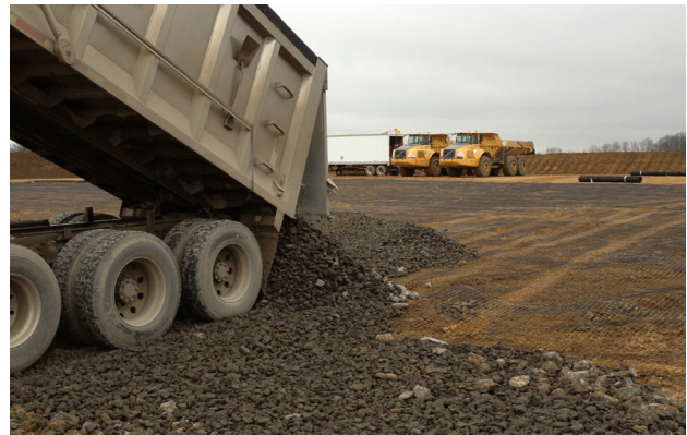
Tensar® TriAx® Geogrid was installed at the Warner and Bame well pad sites to stabilize soft soils.
