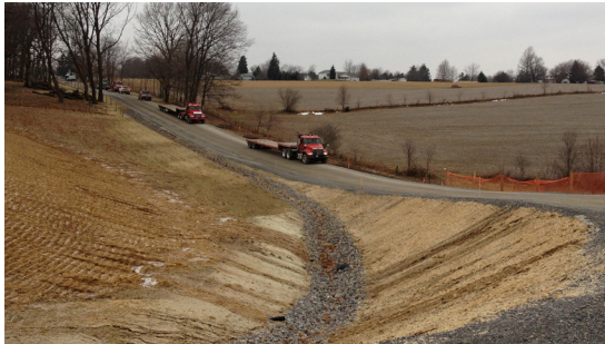
TriAx Geogrid proved to be extremely effective in stabilizing soft soils for the Rex Energy well pads and access roads.
