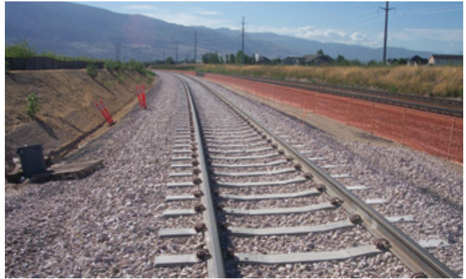
By using Tensar's Geogrid the Utah Transit Authority had significant reduction in material and labor costs.
