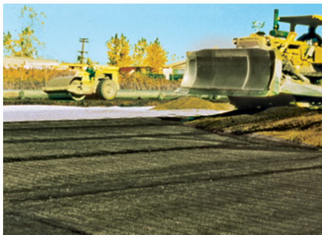
Installation of geogrid at the Canadian Pacific Railway facility in Detroit, MI.
