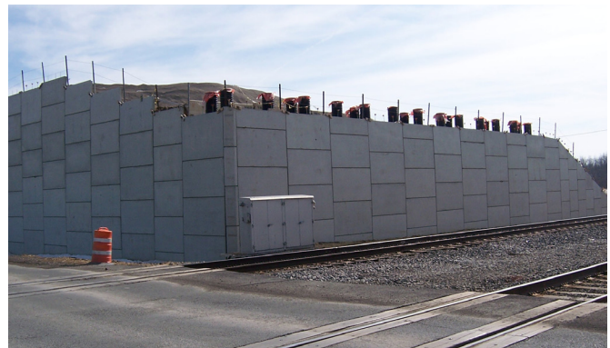
Double rows of tightly spaced piles support the abutments for the Delaware County Road 124 bridge over a CSX railway line.
