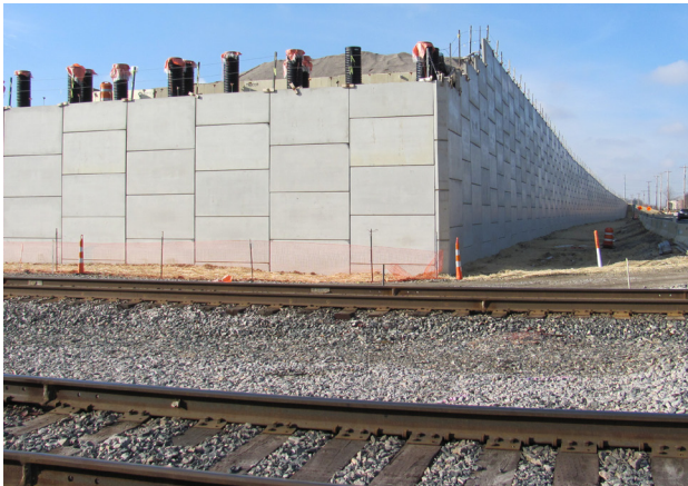
A specified plain smooth form finish for the MSE retaining wall panels left little room for error caused by panel damage or misalignment.
