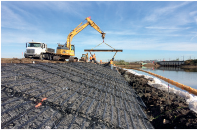
The mattresses were lifted off the delivery truck and directly placed on the embankment.
