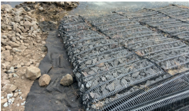
Two mattresses were specifically created in a trapezoidal shape to fit with the site's unusual contours.
