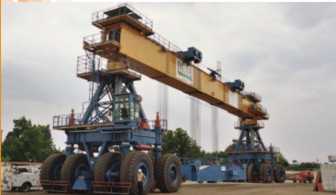
The yard’s ‘driveways’ were designed for this custom-engineered 300-ton straddle carrier which lifted, transported and placed 452 wing-shaped precast bridge segments at the facility.
