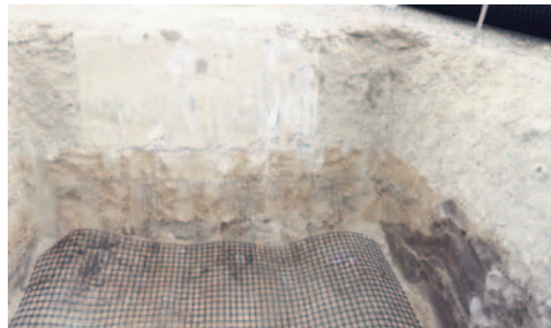
Structural fill beneath the 4-ft-wide shallow spread footing was reinforced with two layers of Tensar® BX1200 Geogrid.
