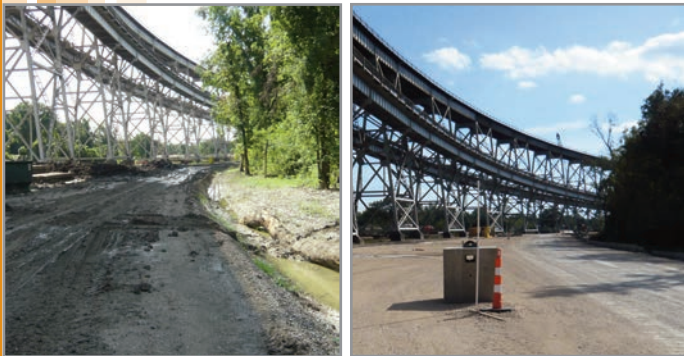
Unimproved (left) versus improved/reinforced (right) working surfaces adjacent to the east bank superstructure.
