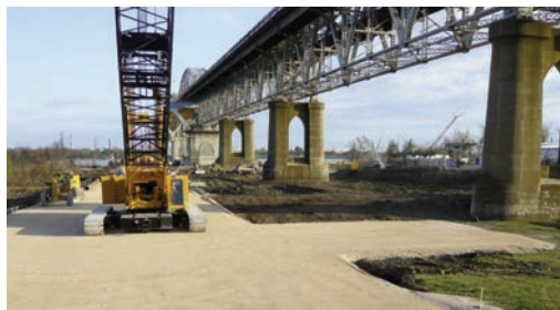
A Manitowoc 2250 crawler crane maneuvers for a pick on the west bank access road/pad.
