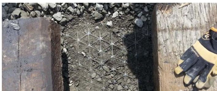
The geogrid was examined 9 months after installation and was still performing as designed.
