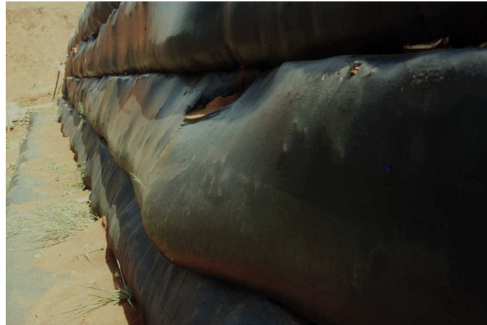
Figure 7: Damage to a woven PP geotextile due to excessive exposure to UV (sunlight) in Indonesia
