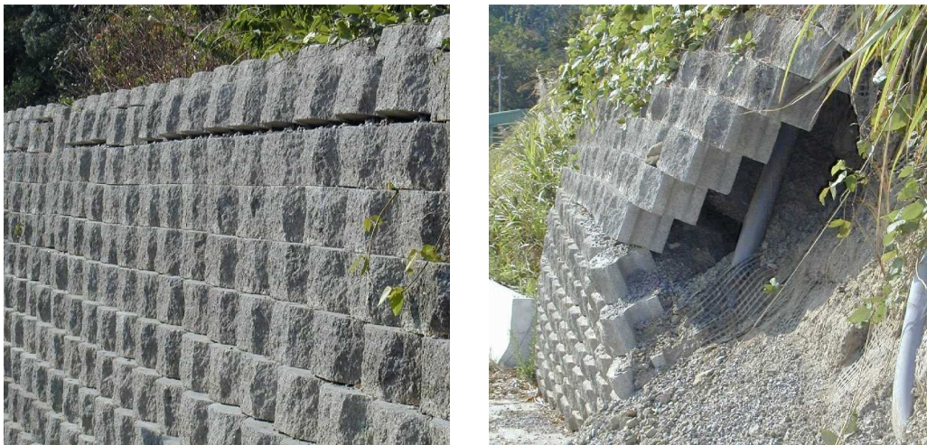
Figure 1. Two modular block retaining walls located close to the epicentre of the 1999 Chi Chi earthquake in Taiwan, showing the results of strong shaking (Site 3 on left, Site 1 on right)
