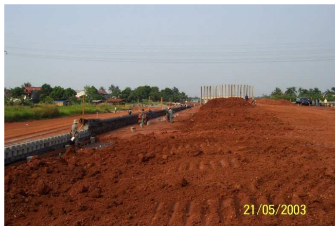
Figure 2: Using tanah merah in the construction of the Jakarta Outer Ring Road
