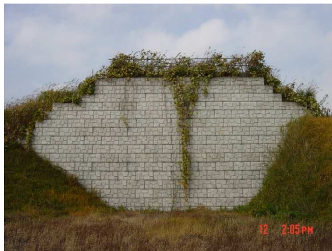
Figure 16a: Japanese trial wall 8m high with sand fill (Nakajima et al, 1996)
