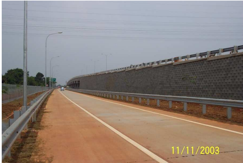
Figure 20: One of the many reinforced soil retaining walls built using clay as part of the Jakarta Outer Ring Road
