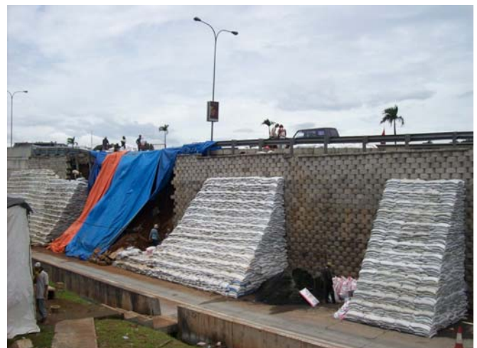
Plate 2 Jalan Veteran MBW facing failure
